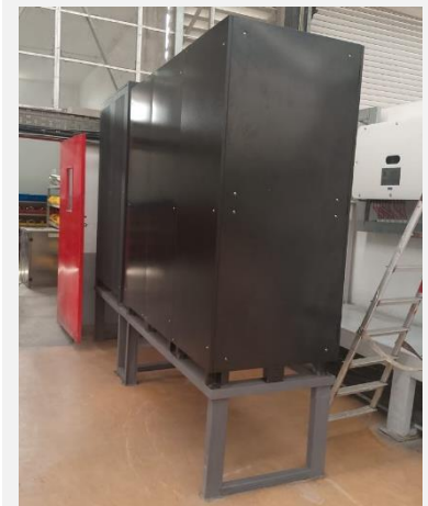
■ Uninterrupted power system (UPS) prevents power disruptions from affecting operations
