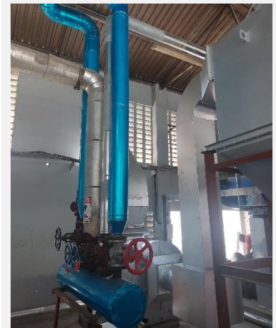
■ New lagging and cladding on the steam line is reducing radiant heat loss on the pipes
